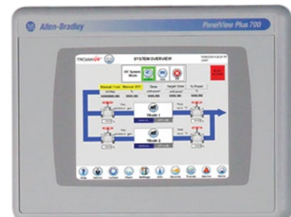
The PLC-based controller combines sophisticated system operation and reporting with an operator-friendly, touchscreen display.
