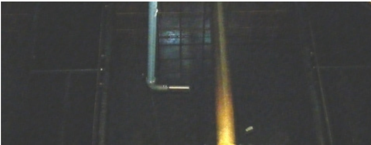
Figure 1. Solitax solids/turbidity sensor installed 12 inches above filter media at the Town of Bethlehem Water Treatment Plant. Solitax is located between the two backwash troughs facing the flow toward the left trough.
