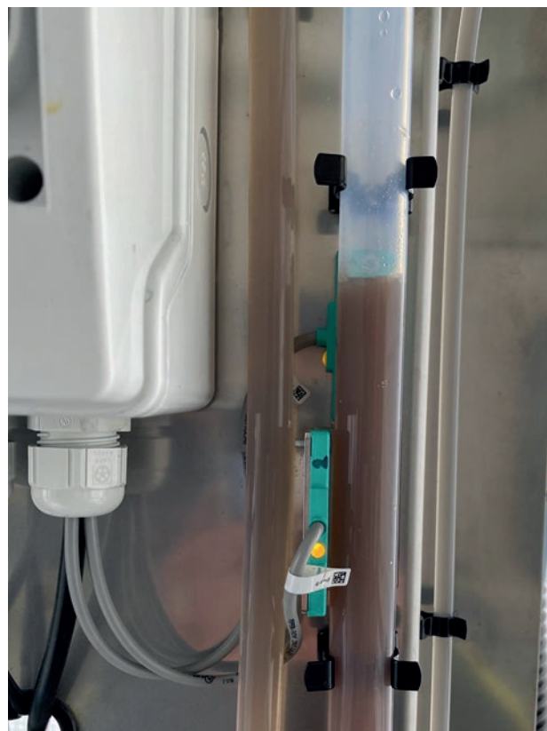
No clogging from activated sludge
