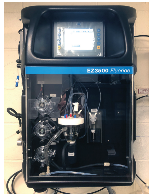
EZ3507 Analyzer installed to monitor fluoride concentration in finished drinking water.
