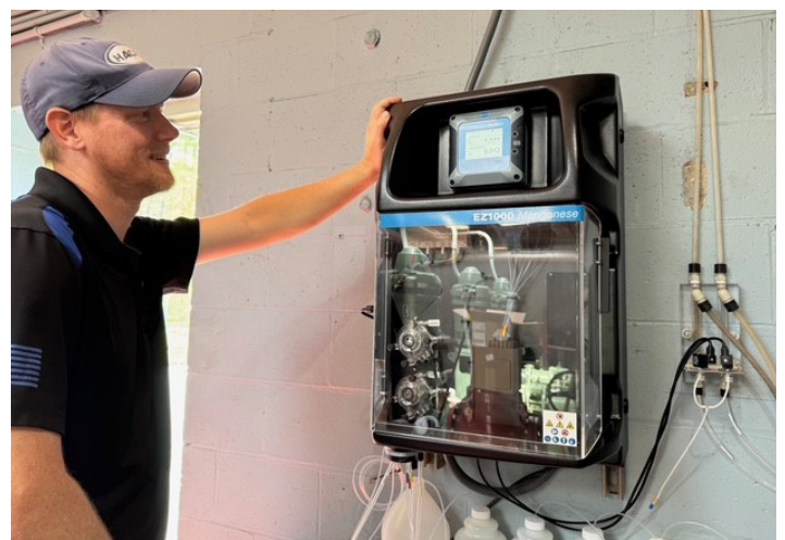
Doug Curtin (Hach Field Service Technician III) maintaining the EZ1025sc 2-Stream Dissolved Manganese Analyzer
