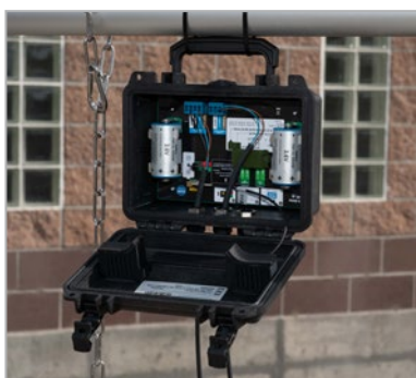
Field Transmitter and cabling
