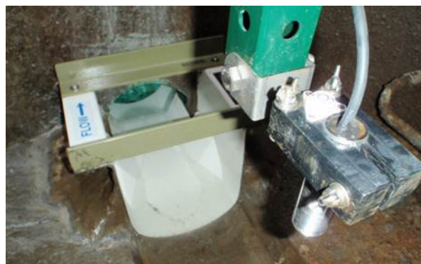
Hach US9001 sensor installed in manhole and measuring the depth of the flow going into an insertion flume
