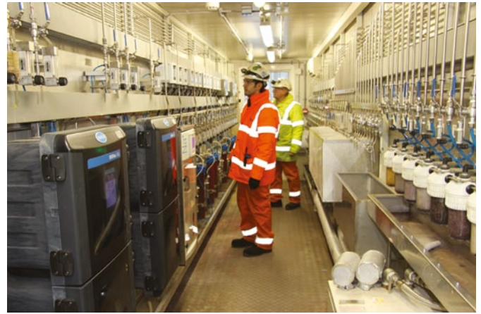
Boiler analyser house
