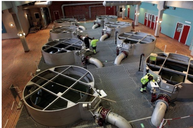
Softening reactors at Vomb waterworks
