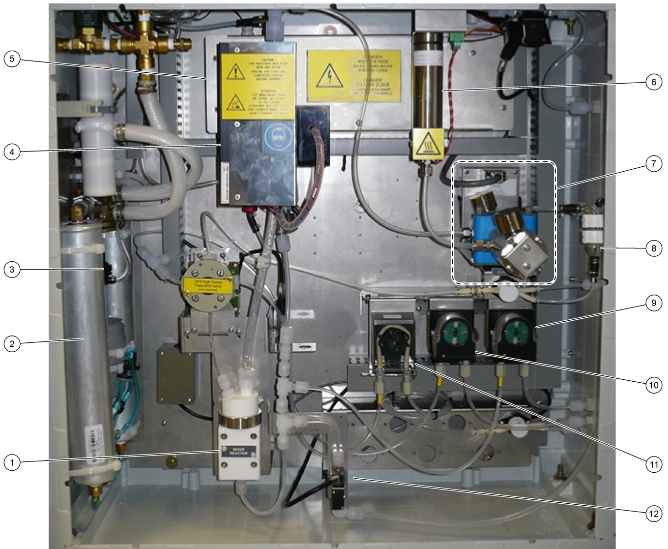
Figure 4 Analysis enclosure—Pumps and components (before September 2022)
