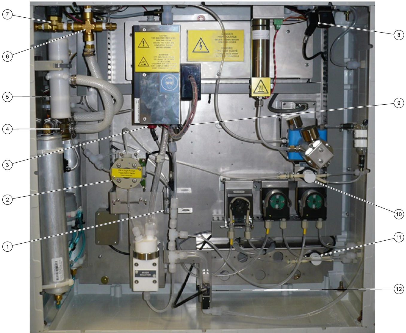
Figure 5 Analysis enclosure—Valves (before September 2022)
