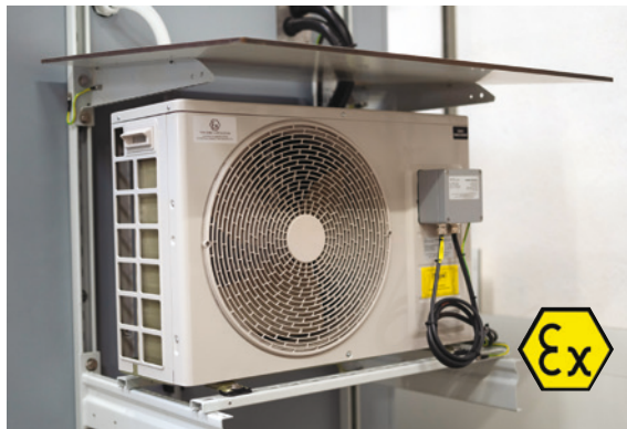
Air conditioning outdoor unit
