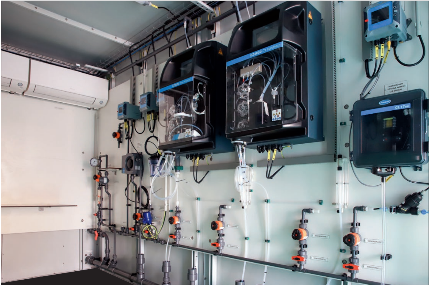
Anashell analyser shelter for Calcium Hardness, Total Alkality and Chlorine analysers, turbidity and pH sensors
