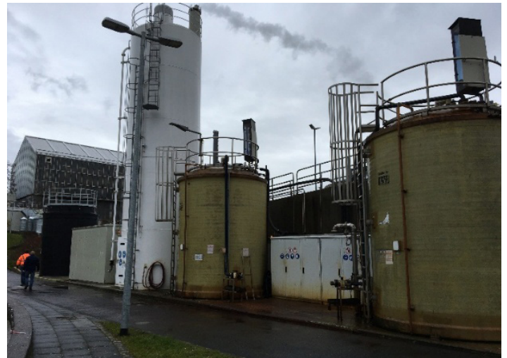
Figure 2: Lime silo and precipitant tanks
