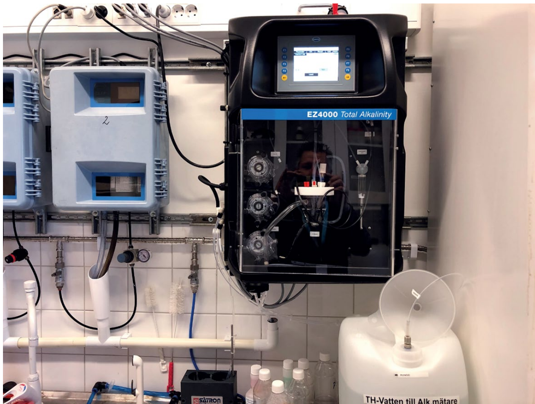
Installation of the EZ4000 Total Alkalinity Analyser at Vomb waterworks
