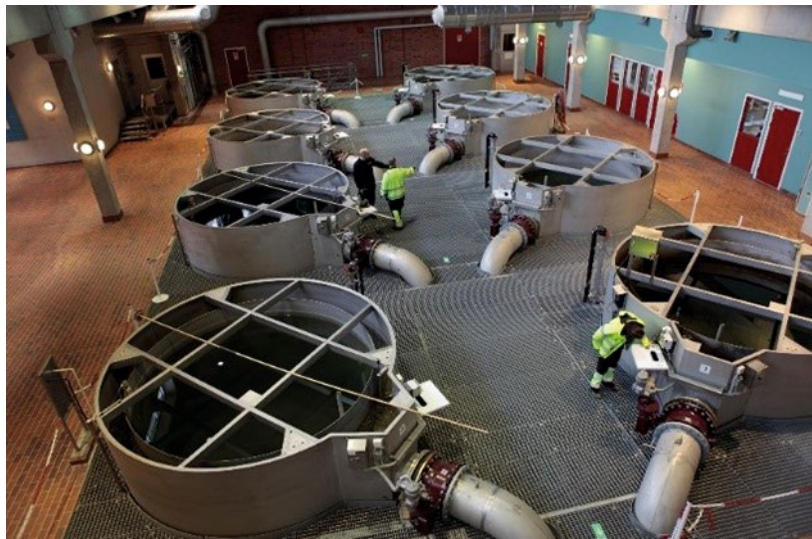
Softening reactors at Vomb waterworks
