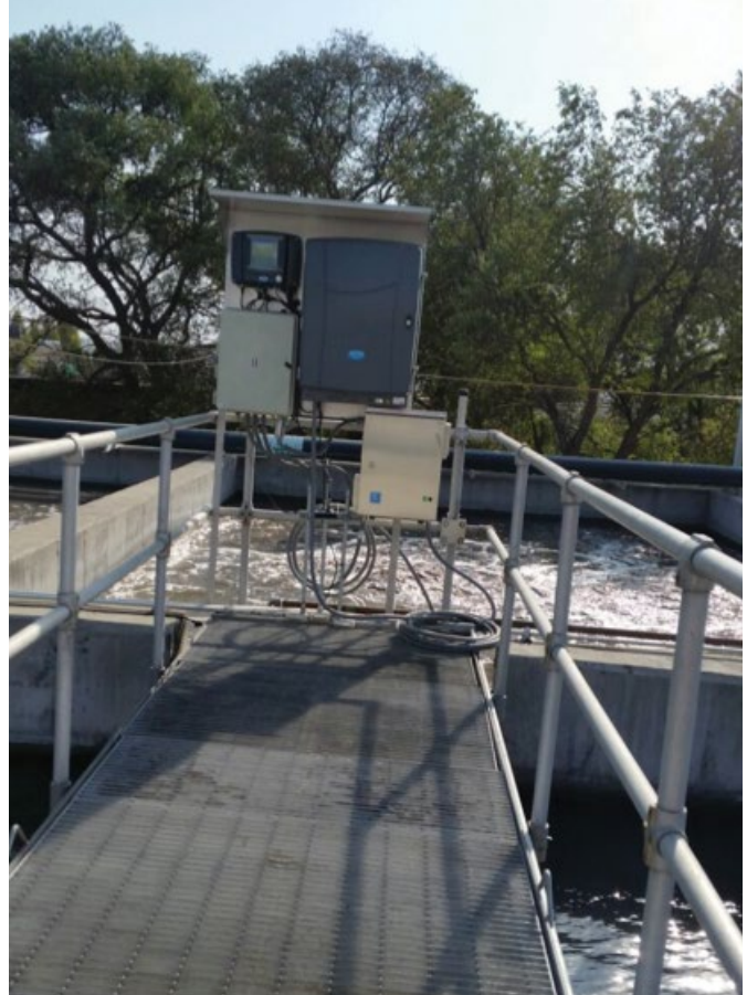
Figure 7: RTC-P installed and running
