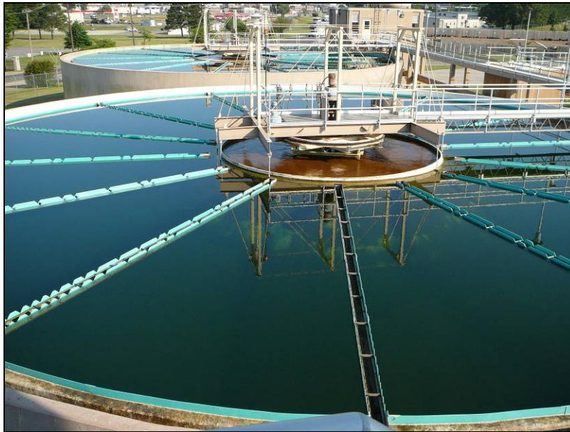
Figure 34: Circular drinking water clarifier with radial launderers and v-notch weir plates Photo by author.
