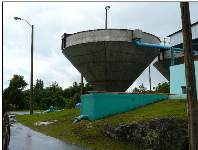
Figure 28: SpiraCone Solids Contact Clarifier Photo by author.
