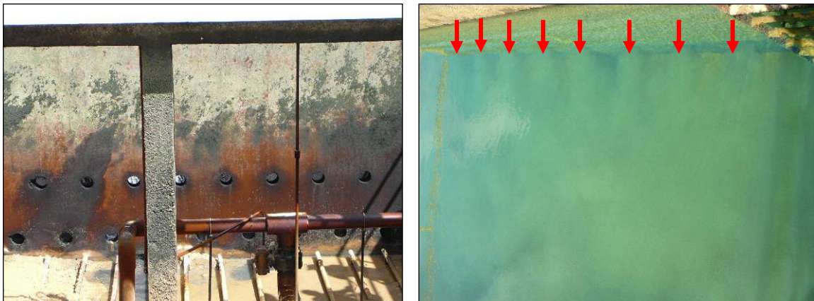
Figure 27: Clarifier w/ perforated inlet baffle wall The rectangular clarifier pictured has a perforated inlet baffle wall. The design is intended to uniformly distribute the flocculated water across the basin to provide uniform settling time and to minimize short circuiting. At left, the perforated inlet wall. Sludge collection pipes (white) visible at the bottom. At right one can see jet streams (red arrows) of the flocculated water entering the basin through the holes. This design would be credited with a baffling factor of 0.7 or better for purposes of calculation of CT. See discussion below under Clarifier Design Impacts Disinfection. Photos by author.
