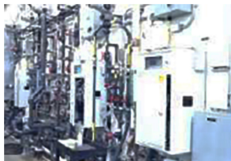
The so-called "Wall of Shame" in a facilities building at Port of Portland featuring the under-performing BIOX units, which have been replaced with Hach BioTector B7000i TOC Analyzers for continuous monitoring of key parameters.
