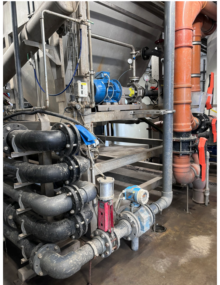
Figure 1: DAF unit of the PreZero process water treatment
