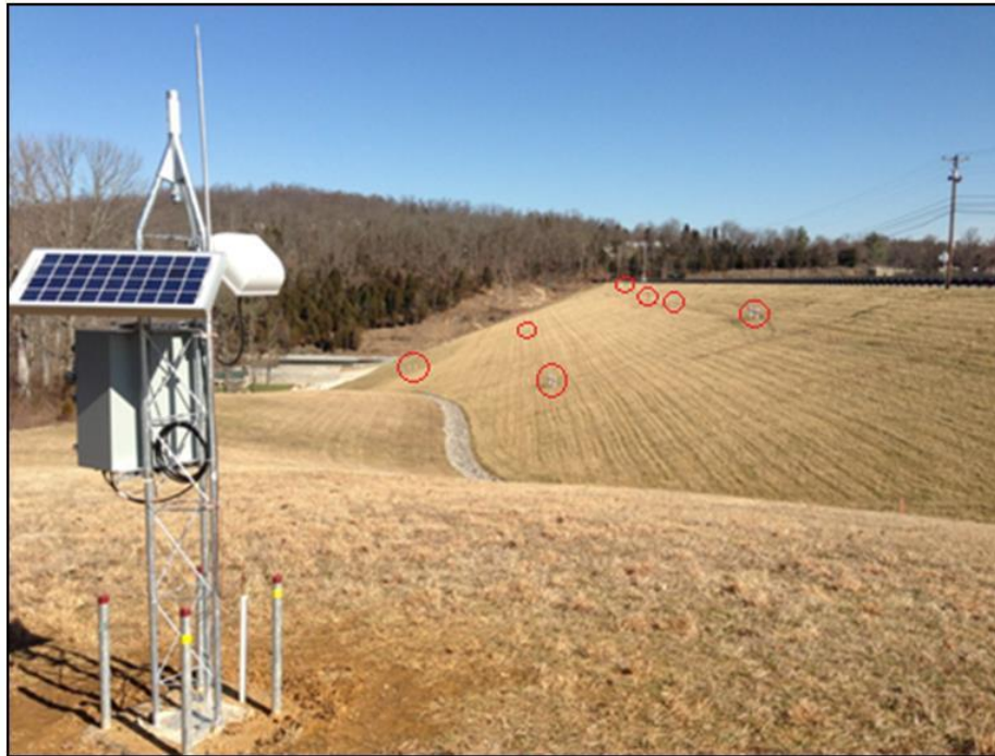
Master Station (Slave stations circled in red)
