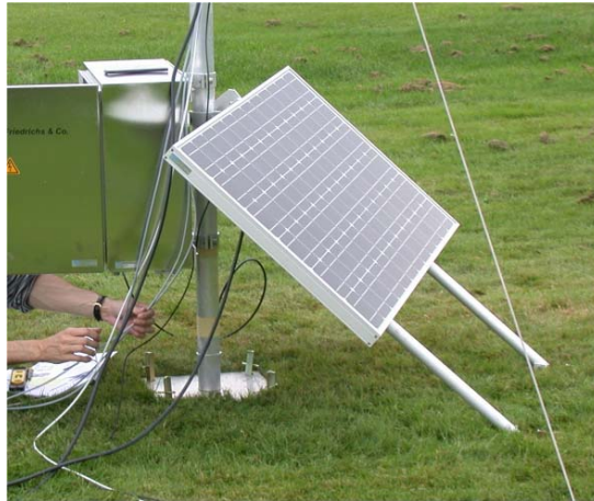
Figure 14: The steel enclosure is fixed to the mast opposite of the solar panel that is facing south (or north on southern hemisphere) and mounted as low as possible in order to leave enough flexibility for the lower temperature sensor. Finally, the wires are led into the enclosure via the cable ducts.
