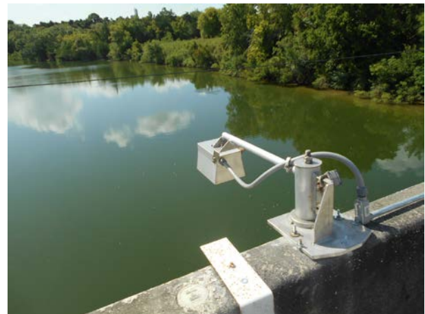
OTT Radar Level Sensor (Photo courtesy of J. Lindner, Harris County Flood Control District)
