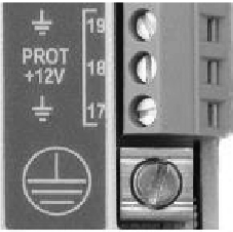
Connection point for earth ground
