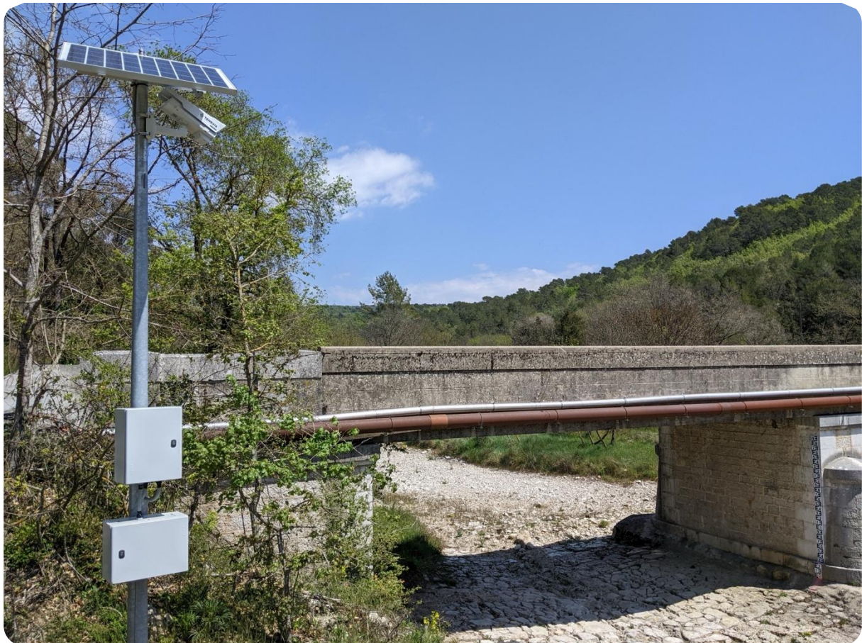
Image 15: HydroSight - Typical measuring site
