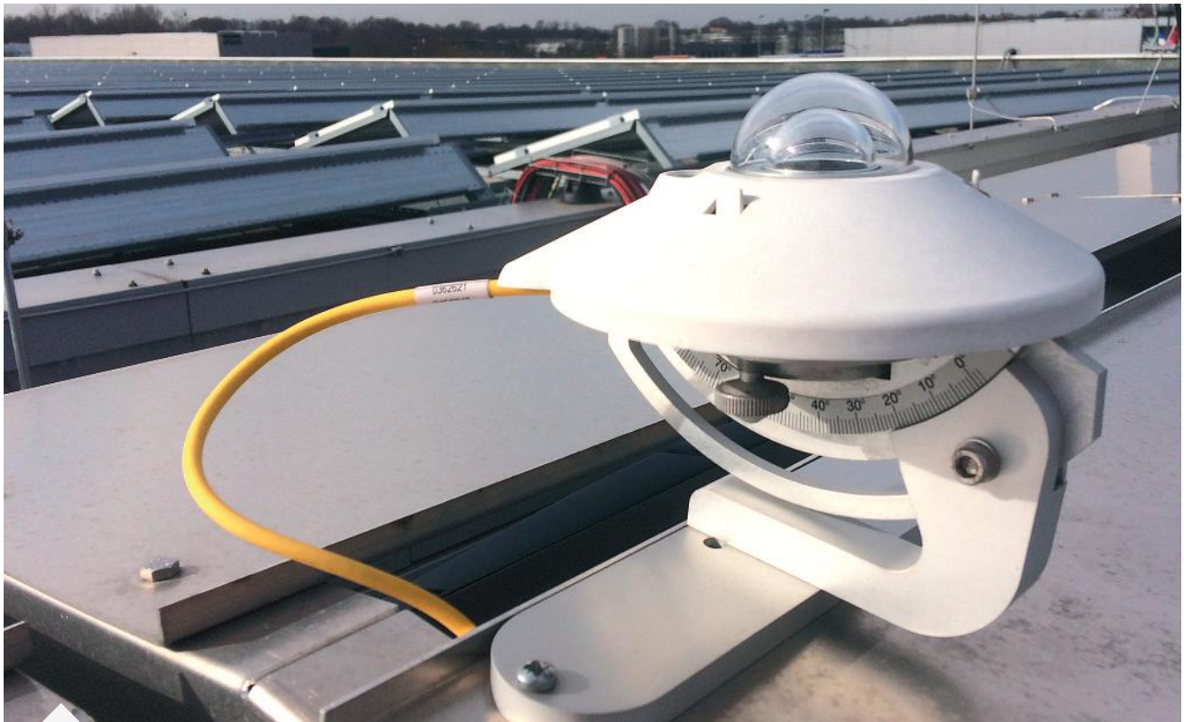
A tilted pyranometer on a roof in Etten-Leur, the Netherlands, a project of SolarAccess Sustainable Energy B.V.
