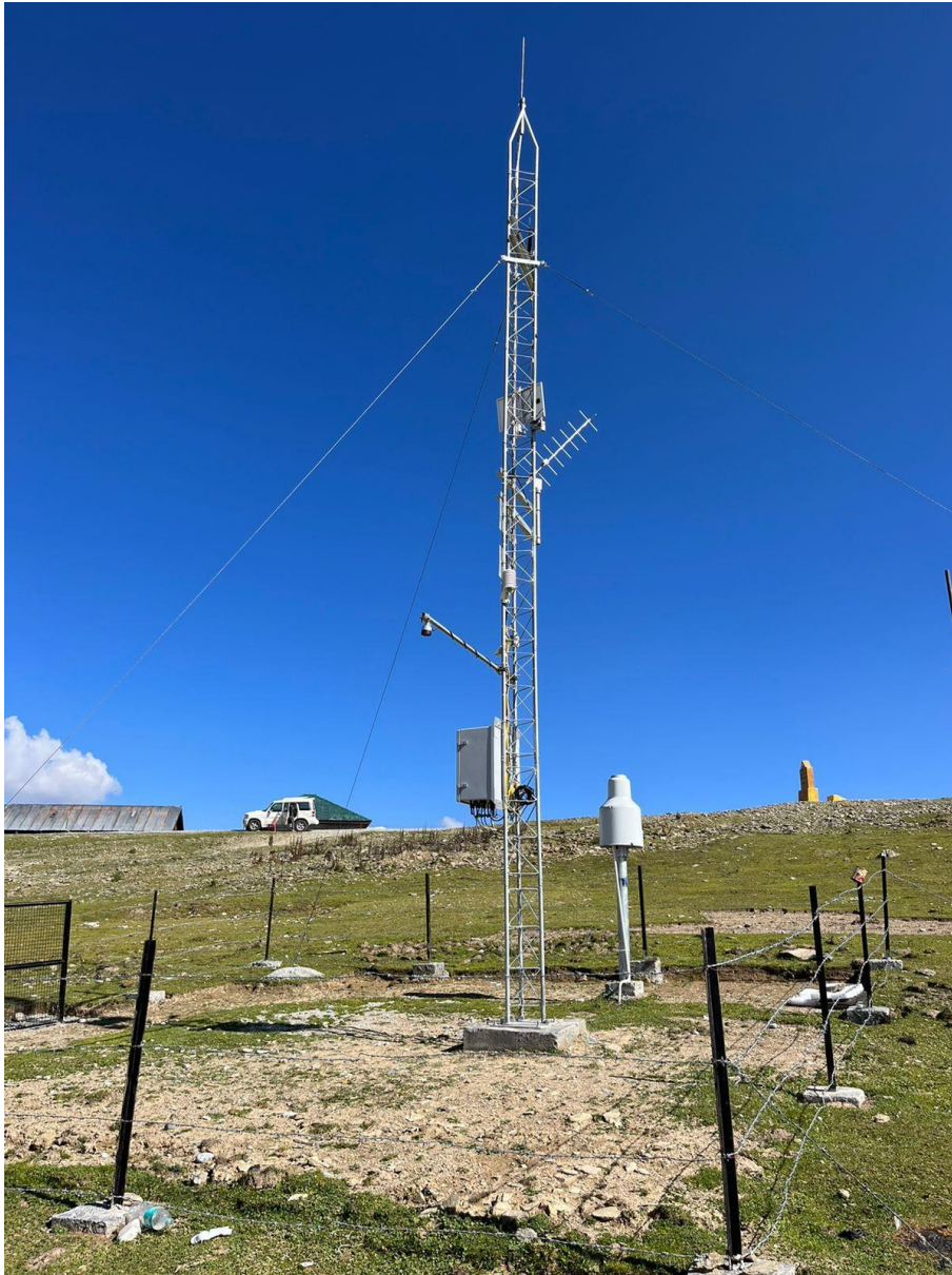
Figure 26. RWIS tower in the field
