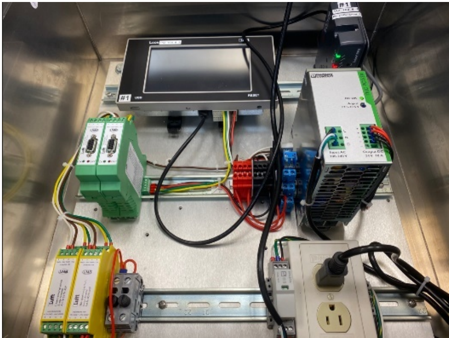
Figure 3. Inside of RWIS enclosure
