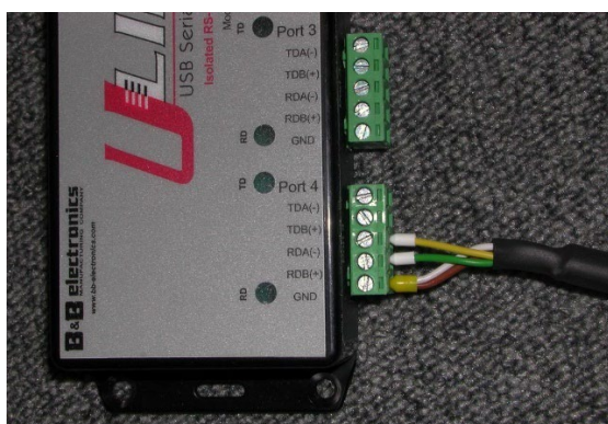
Figure 14 RS485 connection to transducer.
