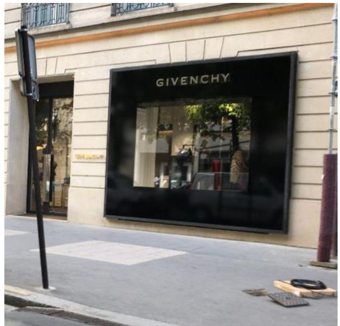
Installation of an ecoLog 1000 monitoring station in the pavement outside of the Givenchy store in Paris.
