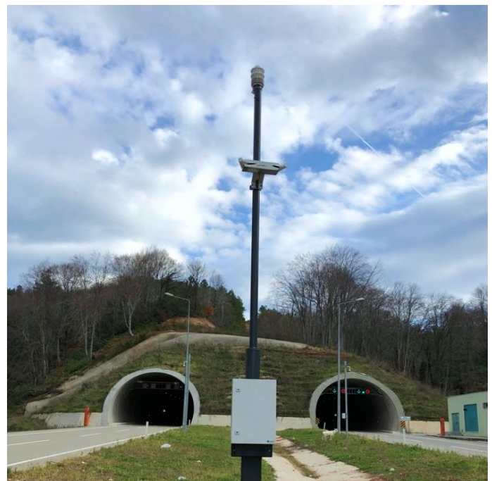
Tunnel station with VS2k, WS600 and IRS31Pro. Photo: WIND İTH.İHR.Ltd.Şti.
